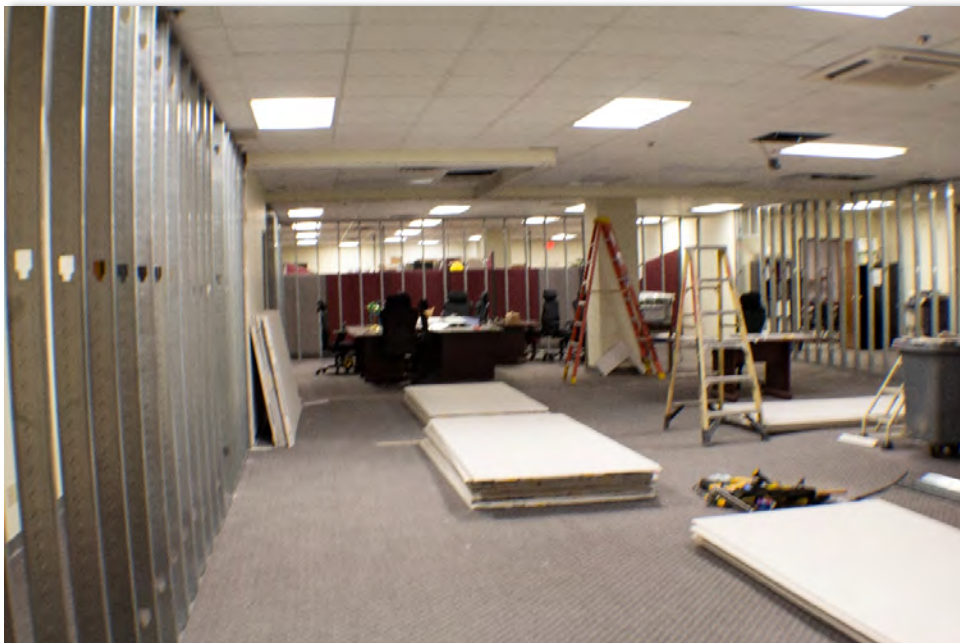
Construction begins on The Justice Center, our in-house learning studio to be completed in FY 2019.
